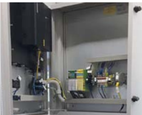
Assembly and wiring
